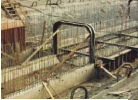
Sea water cooling channels
